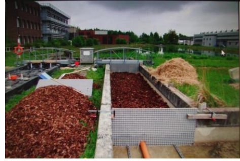
Fig. 2. Picture from the construction site of the “biobed” (photo by Krause Camilo)
